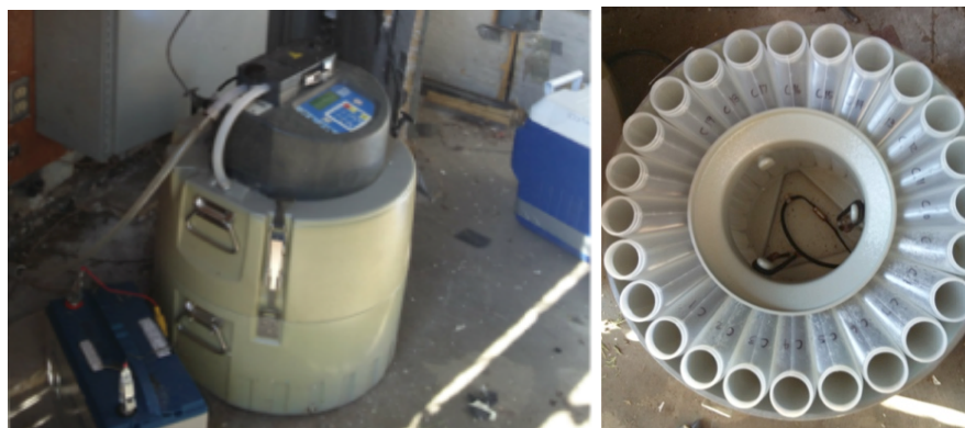
Figure 5. ISCO Model 6712C compact portable sampler and sample bottle carousel installation at the 1300 South stormwater channel site.
